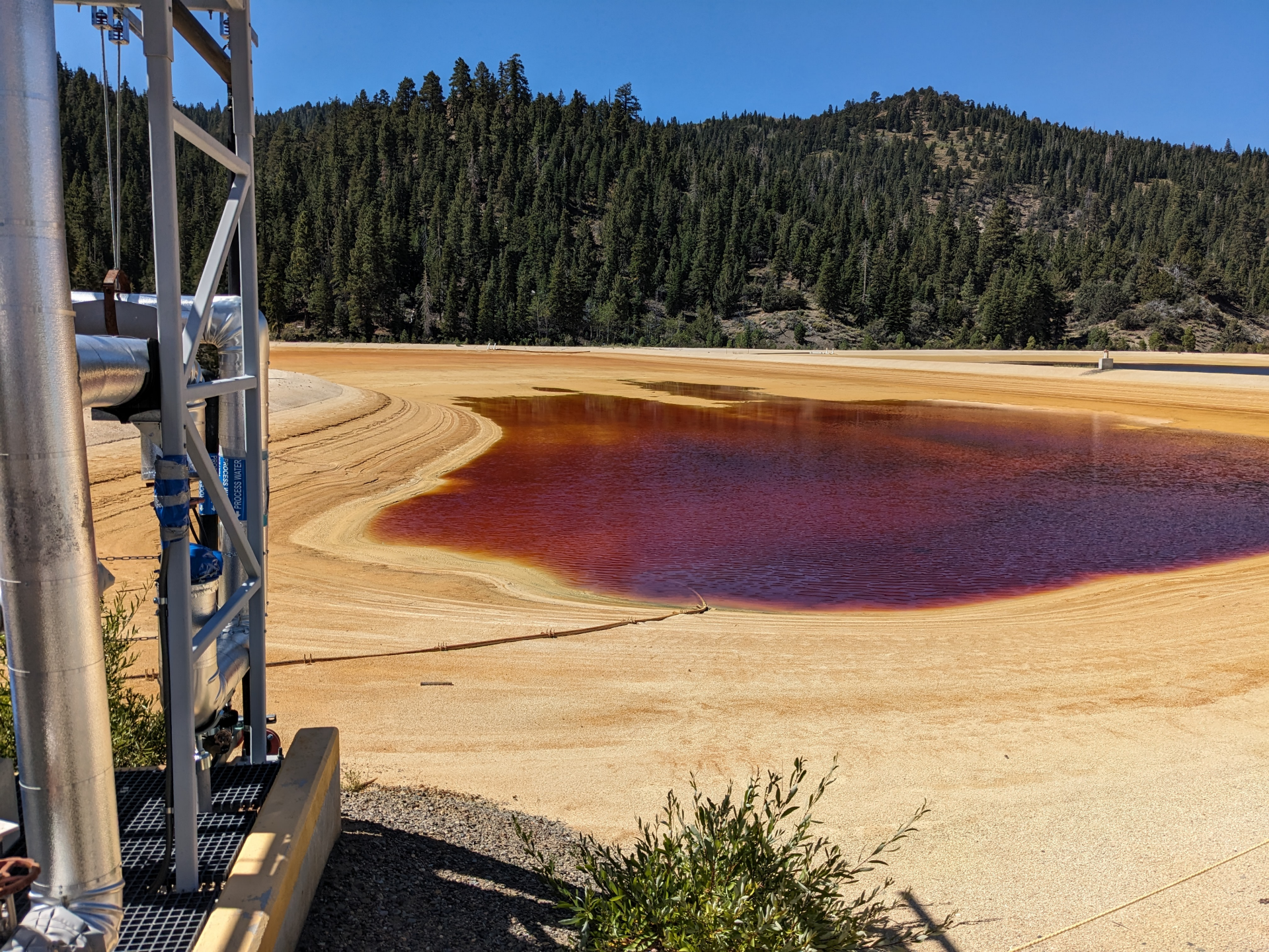
Pond 2 North: part of the pond water treatment system
