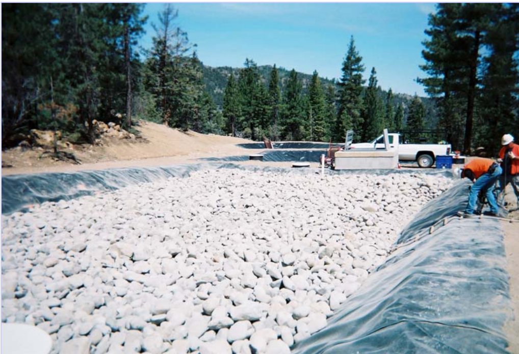
Figure 2: Aspen Seep Bioreactor No. 2 lined with HDPE and filled with river rock.
